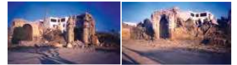
Fig.5 The Compañía Church, Pisco in 2007 after the earthquake: a) Area of the main façade and the entrance to the school, already separated from the rest of the wall pre-earthquake; b) Lateral façade also with separation cracks (credits: Pedro Hurtado Valdez, 2007)
