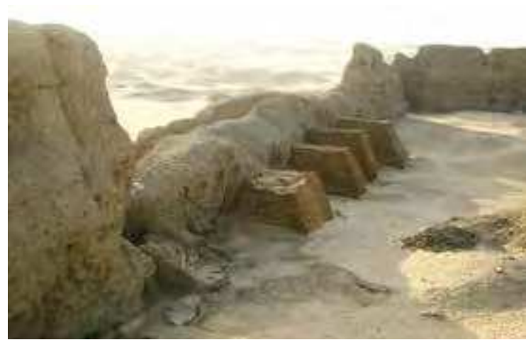
Fig.2 Large sandbag buttresses were constructed in 2001 to support the east enclosure wall (credits: Anthony Crosby, 2006)
