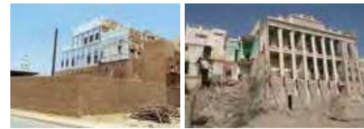
Fig.4 Dar Dawil, the oldest building in al-'Ishshah complex, during restoration (credits: Mohammad al-Junied, 2011)
