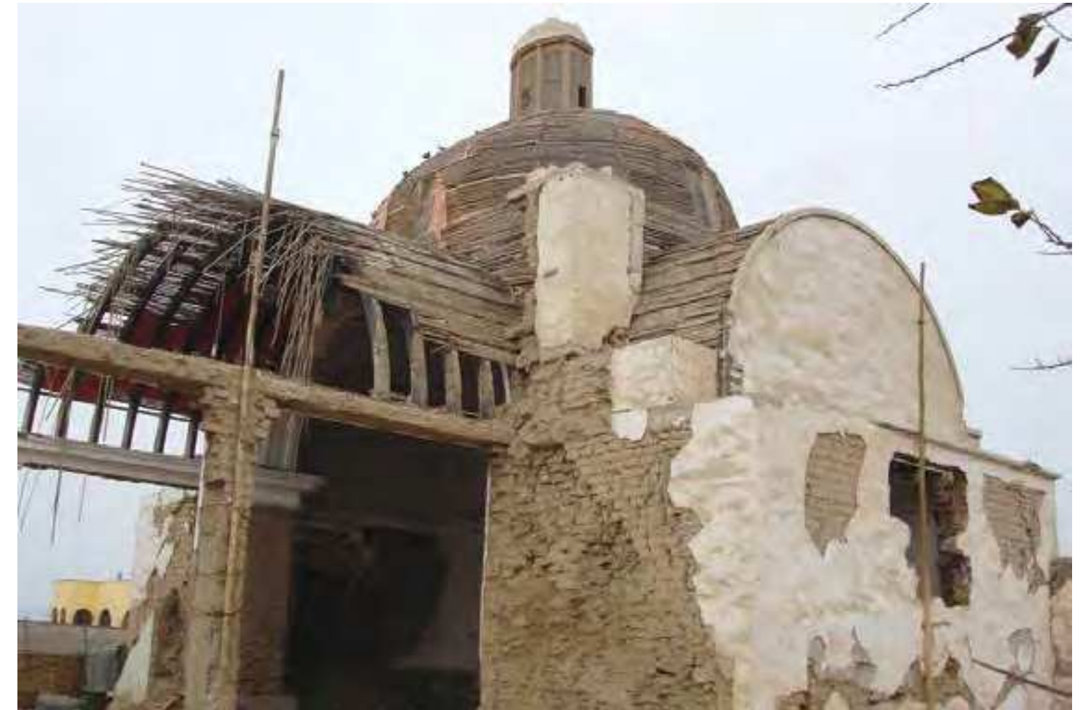
Fig.5 Avoid strengthening with reinforced concrete beams and columns, because they aid in collapse instead of protecting adobe walls, as in this example of the church of San Luis de Canete, damaged during the Pisco earthquake in 2007 (credits: J. Vargas-Neumann, 2007)
