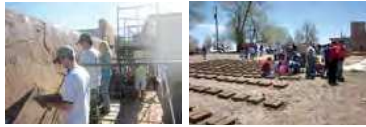
Fig.3 Volunteers plastering walls at San Miguel Chapel in Santa Fe, NM (credits: Jake Barrow, 2011)
