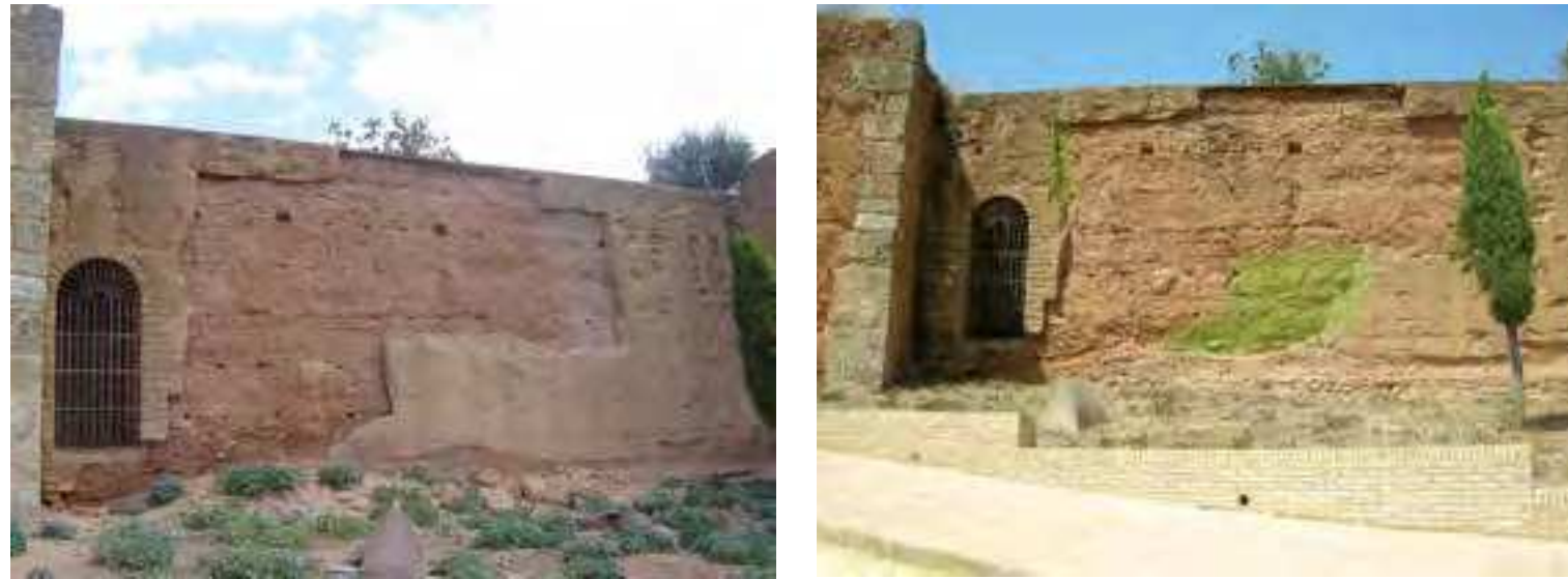
Fig.3 Damage in earthen the fabric of the wall between Towers 6 and 7 in 2009 (credits: A. González, 2009) Fig.4 Damage in earthen the fabric of the wall between Towers 6 and 7 in 2011 (credits: J. Canivell, 2011)
