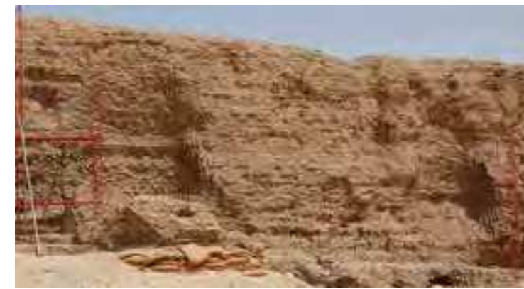
Fig.3 The west enclosure wall showing the completion of the stabilization of two collapsed areas where Coptic cells existed (credits: Anthony Crosby, 2006)
