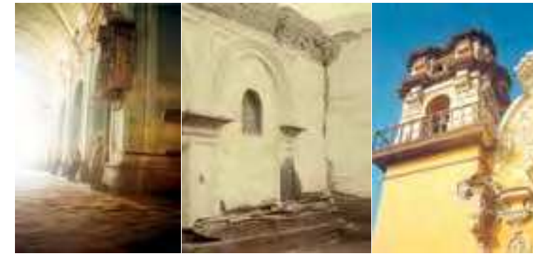
Fig.4 The Compañía Church, Pisco: a) Adobe walls with humidity and differential settlement; b) Adobe walls with loss of the original locking elements and the ties between themselves; c) Crack separating the walls of the tower and façade of the nave (credits: Pedro Hurtado Valdez, 2007)
