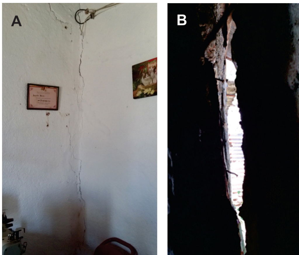
FIGURA 7. A y B) Rajaduras y roturas visibles asociadas al evento sísmico ocurrido el 24 de noviembre del 2016 ( M = 3.4 ) a las 23:29:01.81 hora local (Sánchez Bettucci et al. , 2016b). FIGURE 7. A and B) Visible cracks and breaks associated with the seismic event occurred on November 24th, 2016 ( M = 3.4 ) at 23:29:01.81 local time (Sánchez Bettucci et al. , 2016b).
